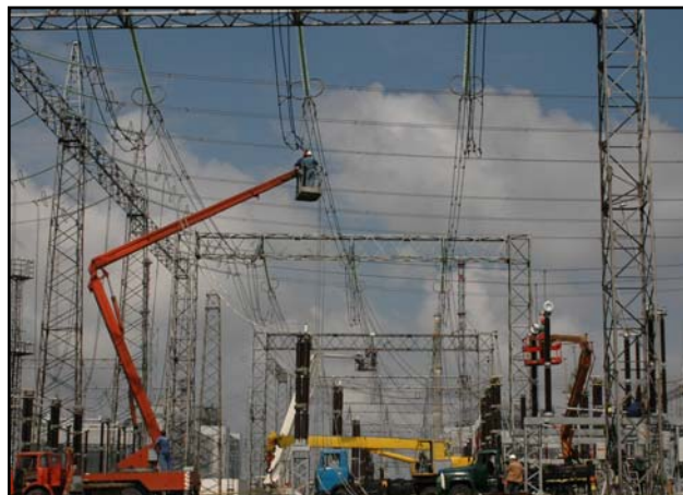
Kozloduy NPP Switch Yard
